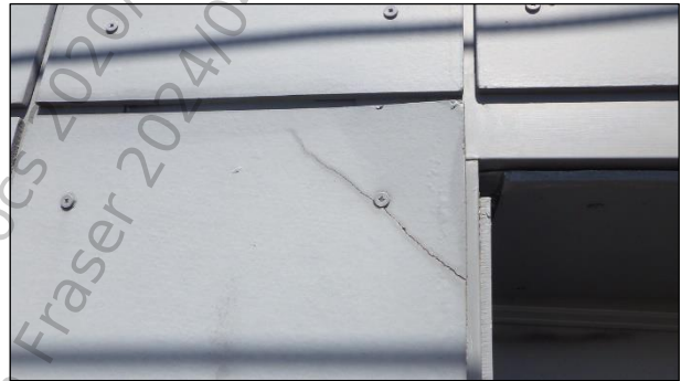
Figure 4 – Cracked panel cladding at rooftop area
