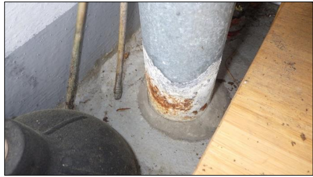
Figure 8 – Corroded metal rainwater leader.
