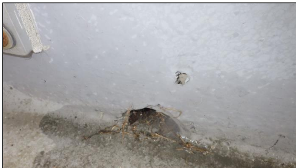
Figure 5 – Discontinuous liquid-applied waterproofing.
