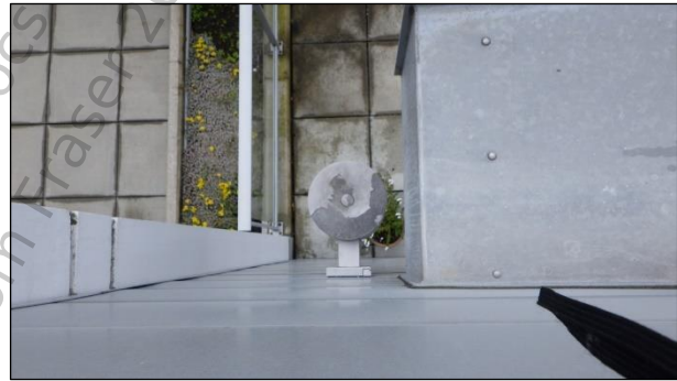
Figure 10 – Deterioration to light fixture paint finish.
