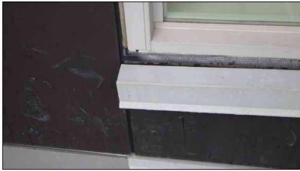
Figure 7 – Detached windowsill flashing
