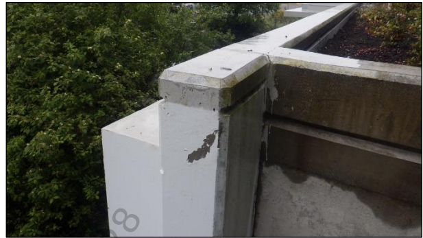
Figure 2 – Failure of wall paint at the parapet areas above the garden suites.
