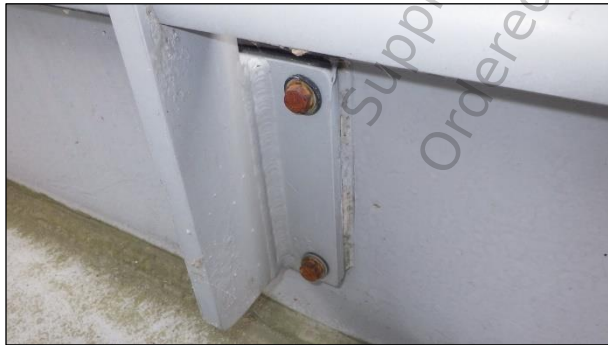
Figure 11 – Corrosion of the guardrail bolt heads. This is mainly a cosmetic issue at this time.
