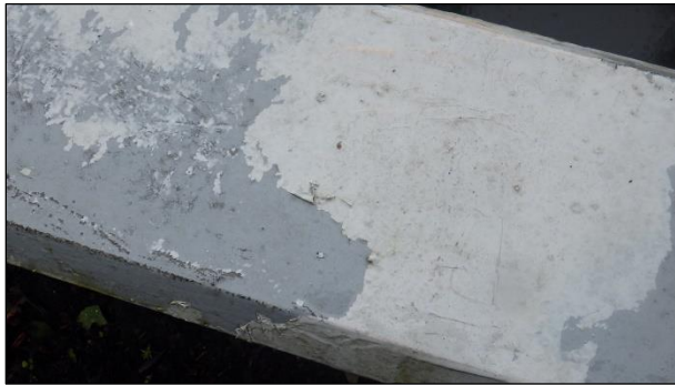
Figure 1 – Failure of liquid urethane waterproofing on the top surfaces of the parapet above the garden suites.
