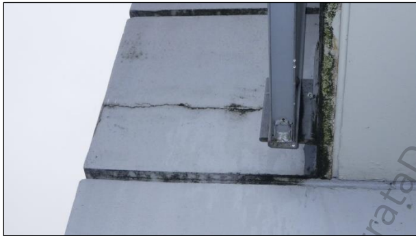
Figure 3 – Hairline cracking, which was noted near various balcony/wall saddles.
