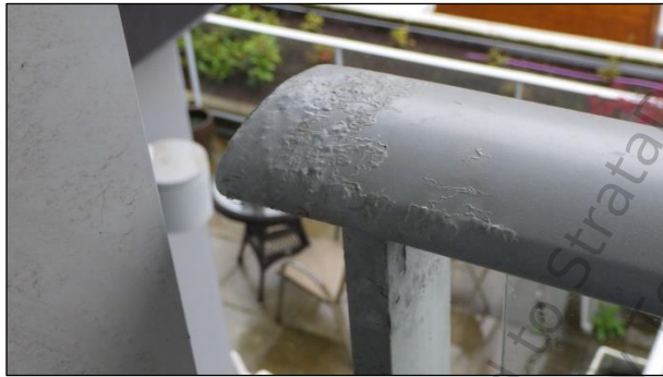
Figure 9 – Guardrail coating deterioration.
