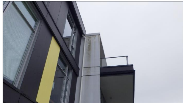
Figure 12 – Staining to wall paint finish.
